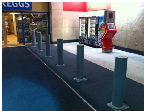
A picture of the finished installation at the shopping centre entrance
