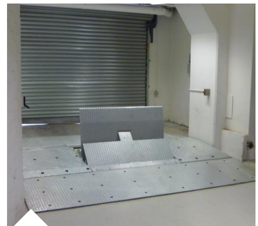
Installed on a suspended slab
